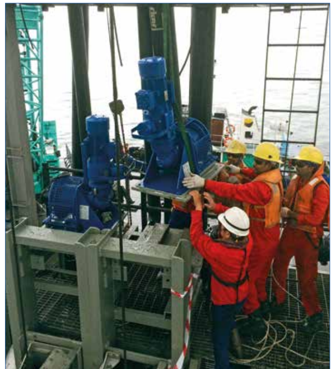
Installation on an oil platform
